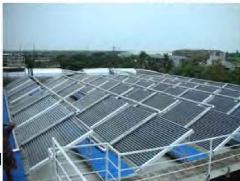
Fig. 8 : Solar hot water installation using tubular receiver in an industry in Gujarat
