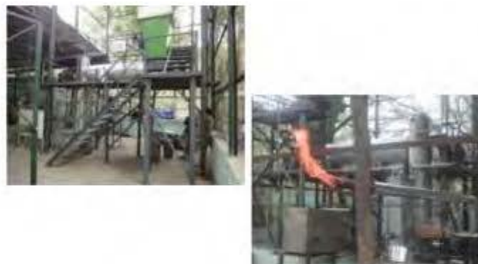
Fig. 20: Two stage gasifier developed at TERI
