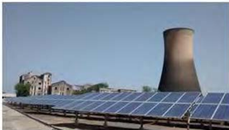
480kW at Shepur, Junagadh
